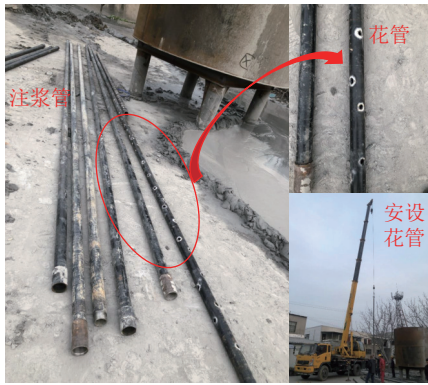
图 3 注浆花管现场安设 Fig.3 Installation of grouting floral tube on site
