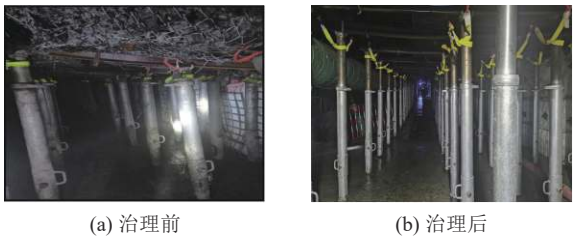
图 18 治理前后遗留煤柱影响区域巷道围岩变形 Fig.18 Surrounding rock deformation of roadway in the area affected by residual coal pillar before and after treatment
